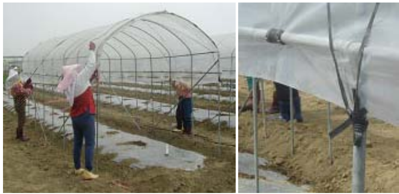
Fig. 8. Plastic sheets are placed over the structure and secured with plastic-wire belts.
